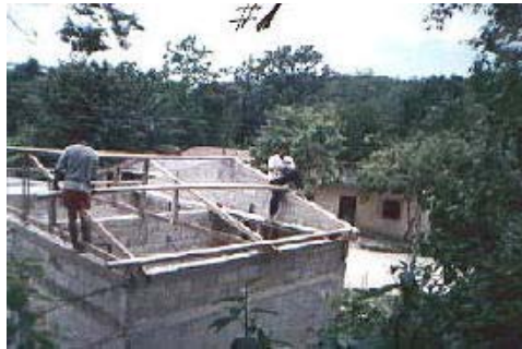
A new roof for a home in the northern Peten region of Guatemala
